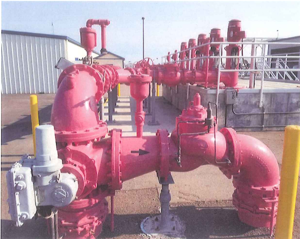
Photo B Discovery Bay Community Service District Sewage Treatment Plant Export Pump Station
