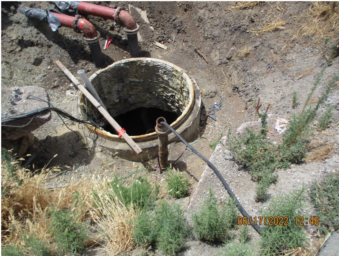
Figure 1 - Pump Station W Currently
