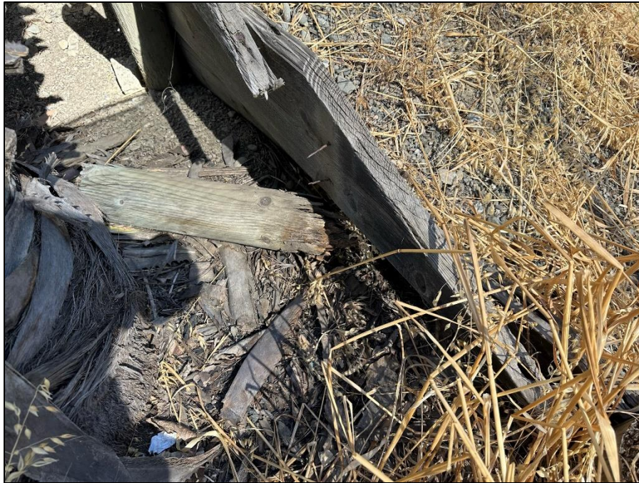
Exhibit 3 – Sheared-Off Wall Post. Rot visible.
