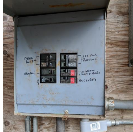
Photo #8 View of outdoor electrical panel for pool equipment
