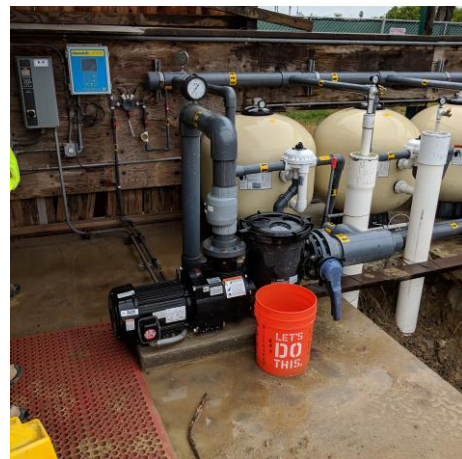
Photo #6 View of existing pump and filters
