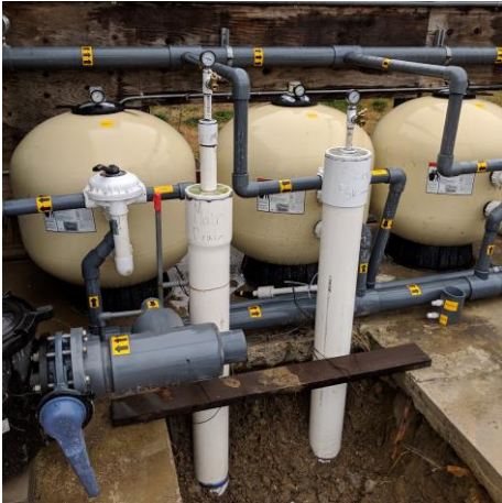
Photo #7 View of filter system
