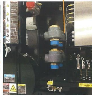
Kunkle Valves (4) Allow cooling air into the vacuum pump
