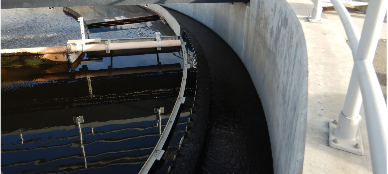
Figure 5: One of the three secondary clarifiers, located at Plant 2, appeared to be in good working condition.
