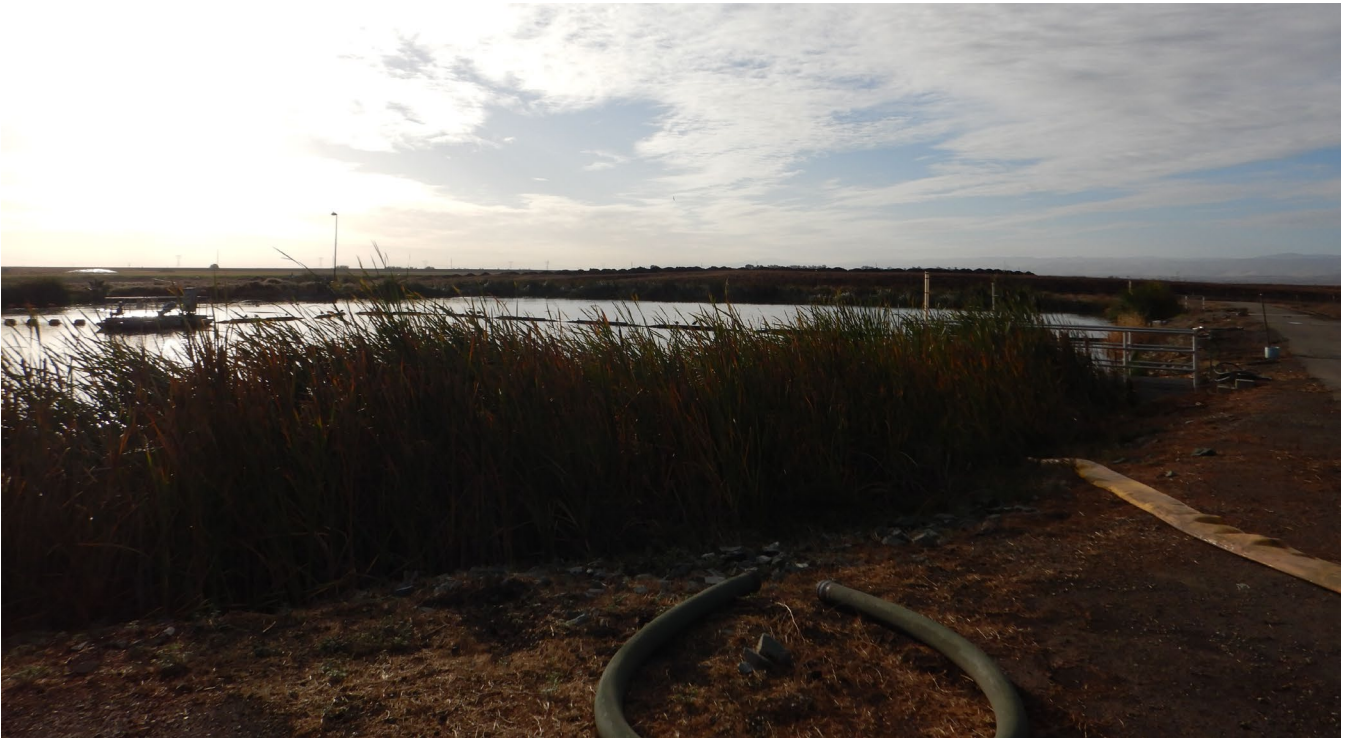
Figure 9: During the inspection, it was observed that storage pond had excessive vegetation.
