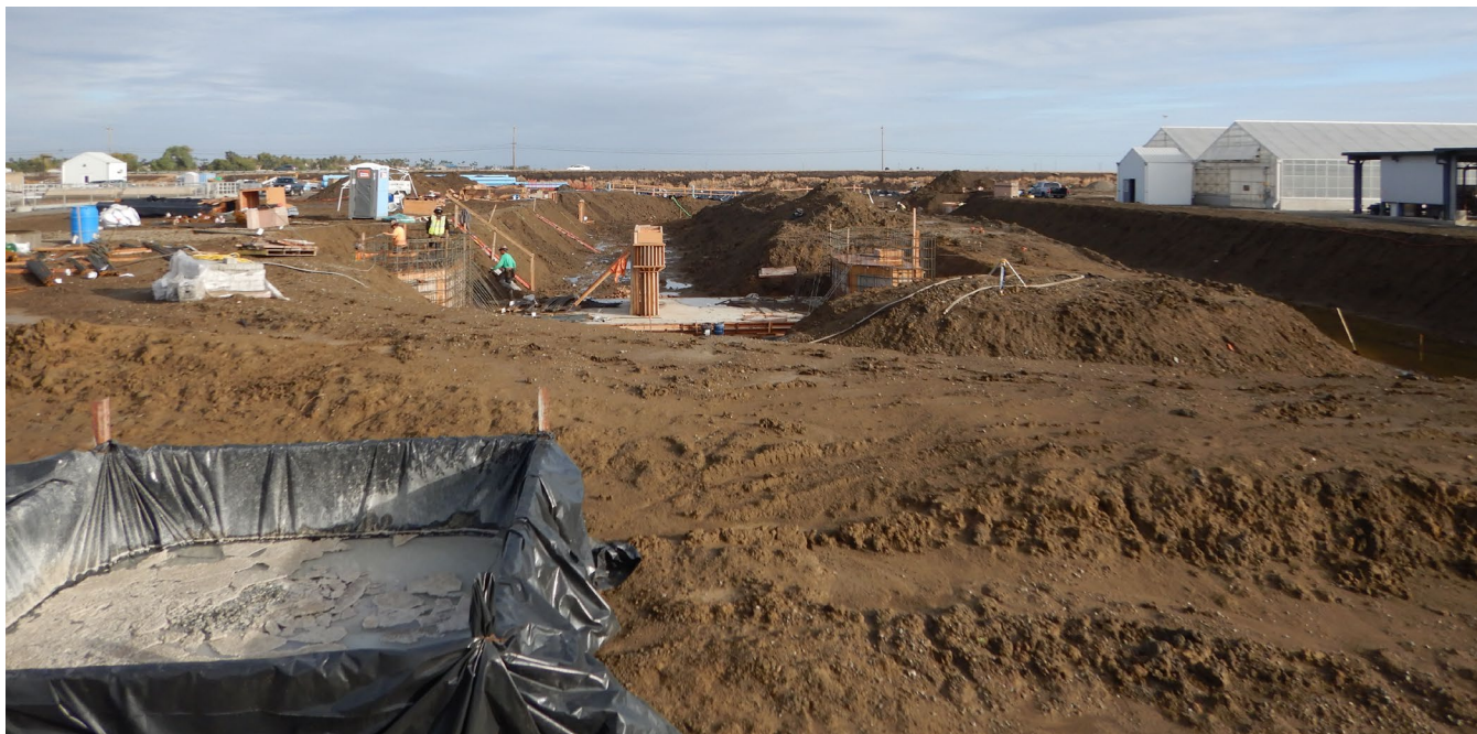
Figure 4: Currently, the Discharger is constructing third oxidation ditch at Plant 2. The Discharger expect to complete the construction activities and bring the oxidation ditch online by early 2023.
