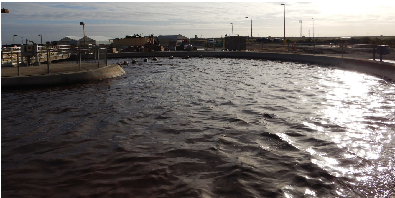
Figure 3: One of the two Oxidation ditches located in Plant 2 appeared in good working condition during the inspection.
