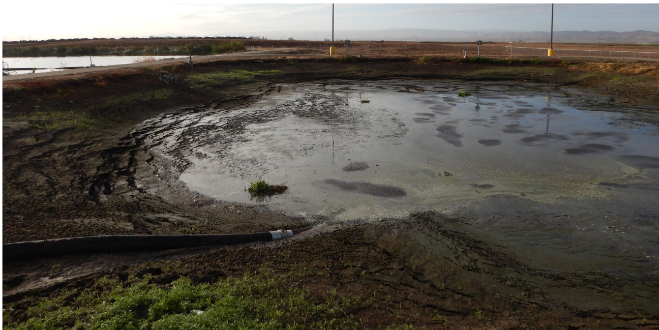
Figure 7: Aerobic digester is out of service for maintenance. Currently, all waste activated sludge (WAS) is discharged to the storage pond.
