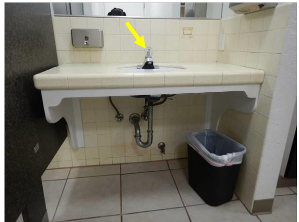
Photo #84 Non-compliant faucet handle in the men's restroom.
