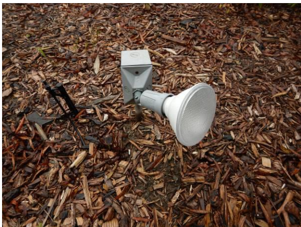
Photo #11 Ground security light fixture.
