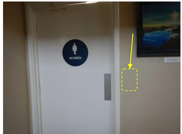
Photo #58 Entrance to women's restroom. Note lack of tactile signage.
