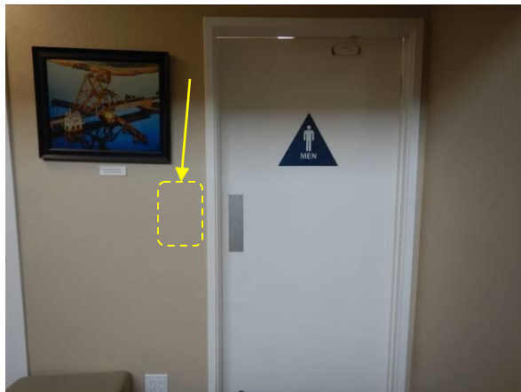
Photo #57 Entrance to men's restroom. Note lack of tactile signage.
