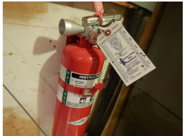
Photo #76 Portable fire extinguishers were observed throughout the property.
