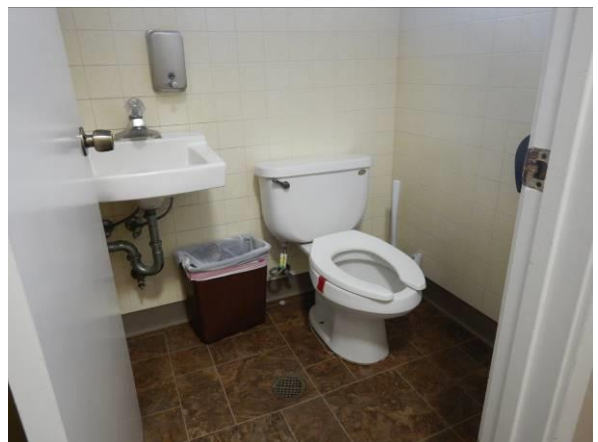
Photo #54 Typical unisex restroom finishes. Note lavatory piping is not protected against contact.
