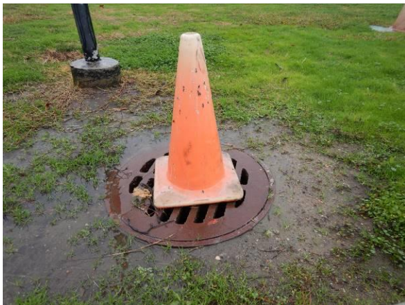
Photo #27 Area drain adjacent to pool area appeared to be clogged at the time of Terracon's site visit.
