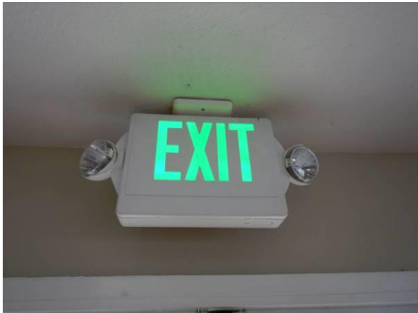
Photo #79 Exit signage is generally provided at exits and along paths of egress.
