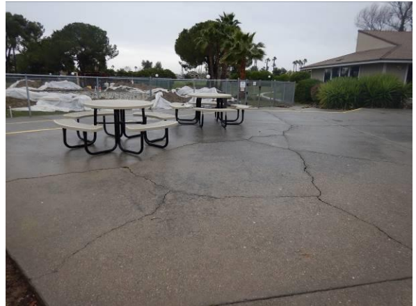
Photo #26 Seating area at east side of building. Note cracking of concrete pavements.
