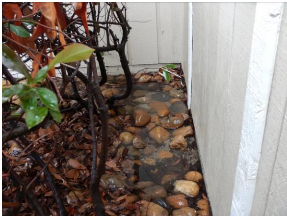
Photo #29 Standing water was observed up against the east side of the building.
