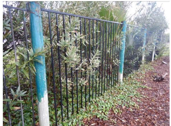
Photo #14 Painted metal fencing with wood posts are provided at limited sections along the west side of the building. Note deteriorated paint.
