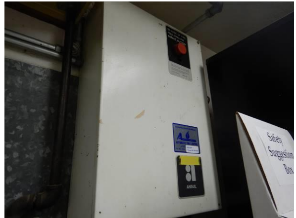
Photo #74 Ansul system.
