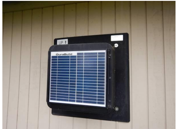
Photo #72 A through-wall, solar-powered fan provides ventilation to the attic.
