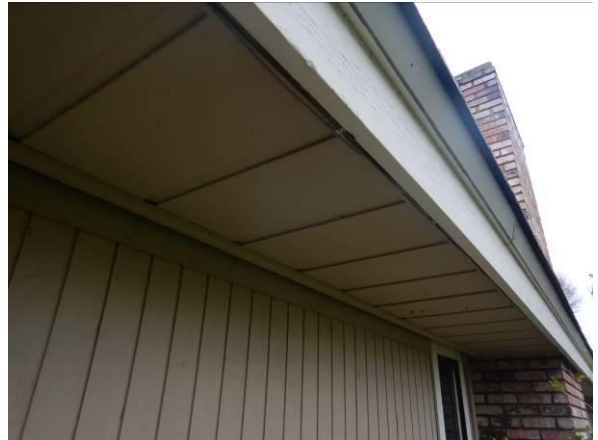
Photo #40 Building exterior walls consist of painted wood siding with metal accents.
