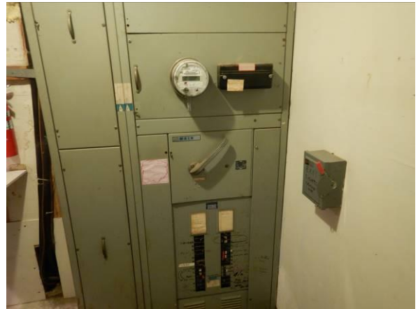
Photo #68 Overview of electric meter and main electrical disconnect switch.
