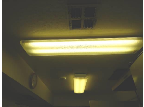
Photo #70 Typical ceiling-mounted fluorescent light fixtures.
