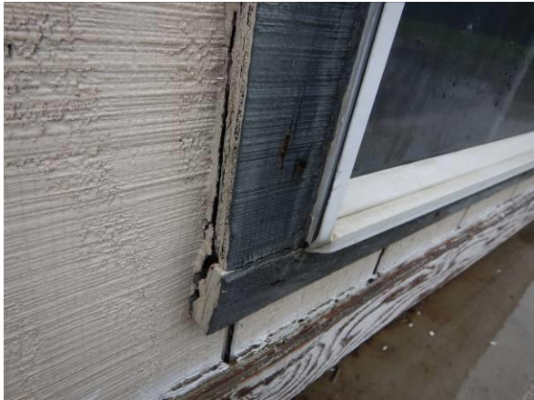
Photo #45 Deteriorated sealants were observed at window penetrations.
