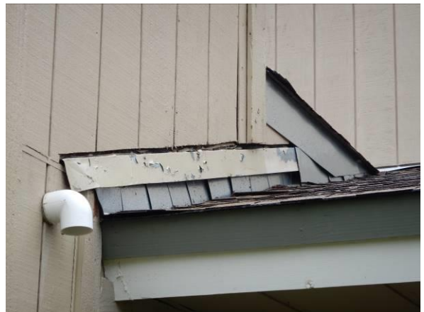
Photo #42 Localized areas of delaminated paint were observed at metal trim and roof flashings.
