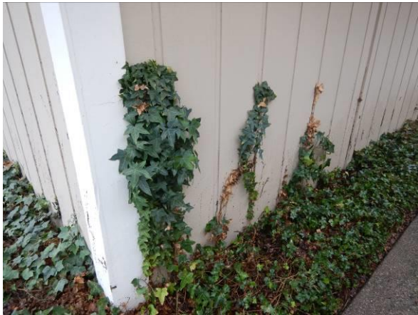
Photo #43 Biological growth was observed at localized areas of the building exterior.
