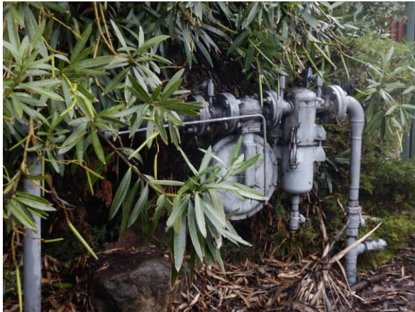
Photo #7 Natural gas meter and service and to the building. Note seismic shutoff provisions are not installed
