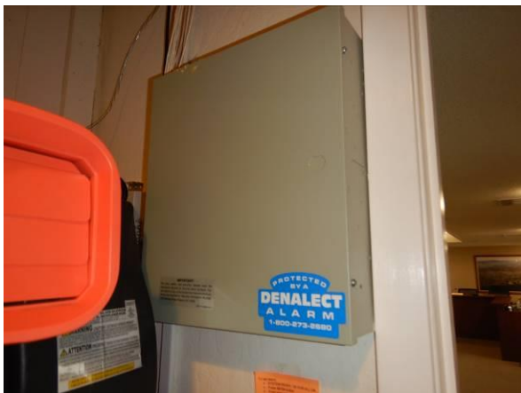
Photo #77 Fire alarm control panel.
