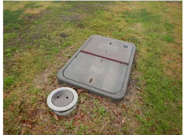
Photo #8 Typical water meter
