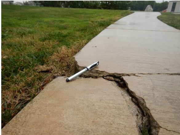
Photo #25 Heaved sections of concrete pavements were observed along the east side of the building. Pen for scale.
