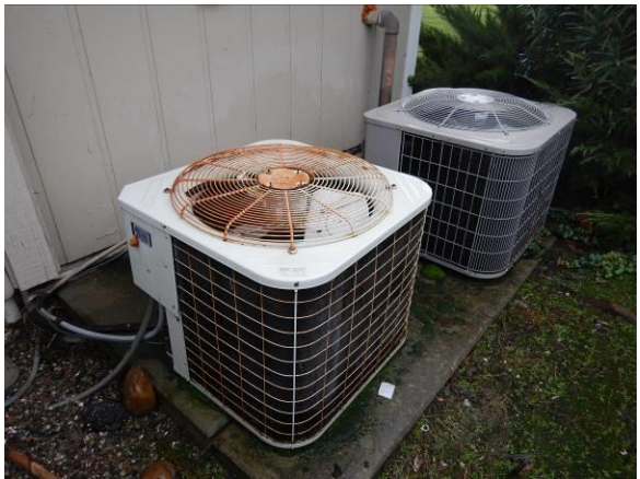
Photo #71 Typical Carrier pad-mounted DX cooling units.
