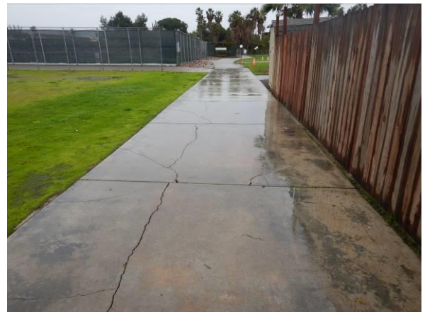
Photo #24 Linear cracking observed at concrete pavements.
