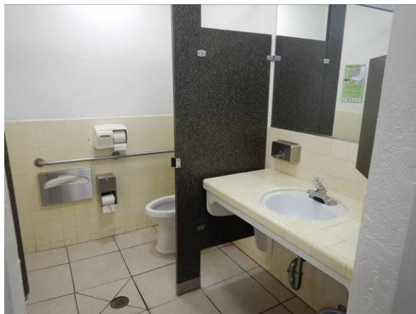
Photo #59 Typical restroom finishes. Note that lavatory piping is not protected against contact. Women's is similar.
