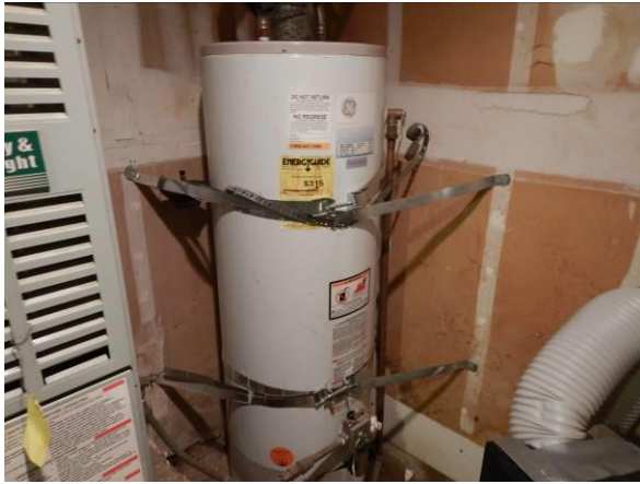
Photo #69 Overview of GE 50-gallon, natural gas-fired water heater.
