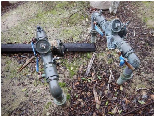
Photo #9 Overview of irrigation control valve
