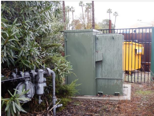
Photo #73 Overview of pad-mounted utility transformer.
