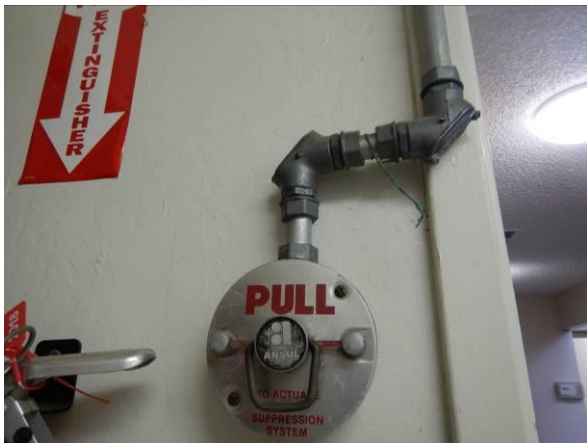
Photo #75 A pull station connected to the Ansul system was observed.
