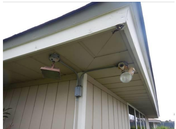
Photo #12 Building-mounted light fixtures.
