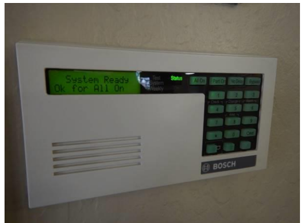
Photo #78 Fire alarm control panel control module.
