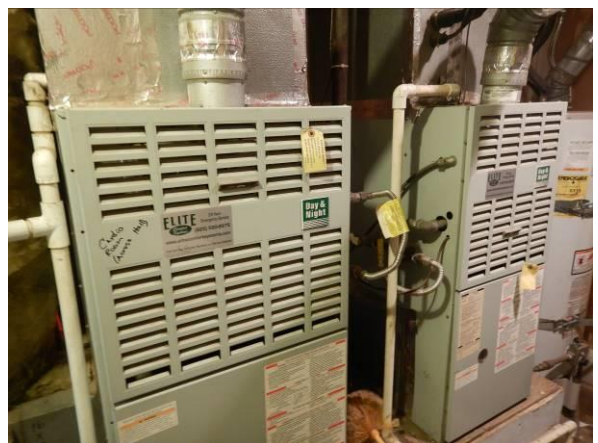
Photo #66 Overview of Day & Night natural gas-fired forced-air furnace located in the electrical room.
