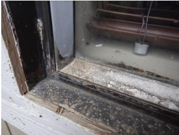
Photo #39 Close-up exterior view of window sill and jamb. Note deterioration of window sealants.
