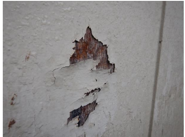
Photo #44 Example of paint damage and deterioration observed in localized areas throughout the building exterior.
