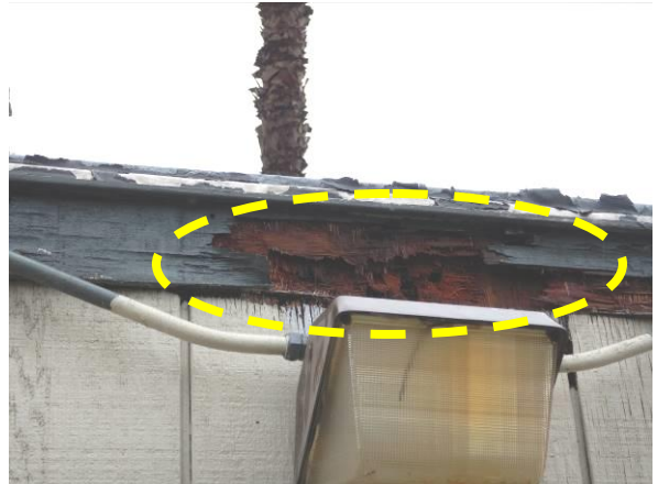
Photo #46 Localized areas of wood decay or otherwise damaged wood trim were observed at the roof edge.
