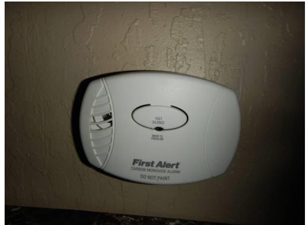
Photo #80 Typical carbon monoxide detector.
