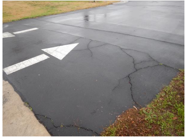
Photo #4 Longitudinal and transverse cracking was observed throughout asphaltic pavements.
