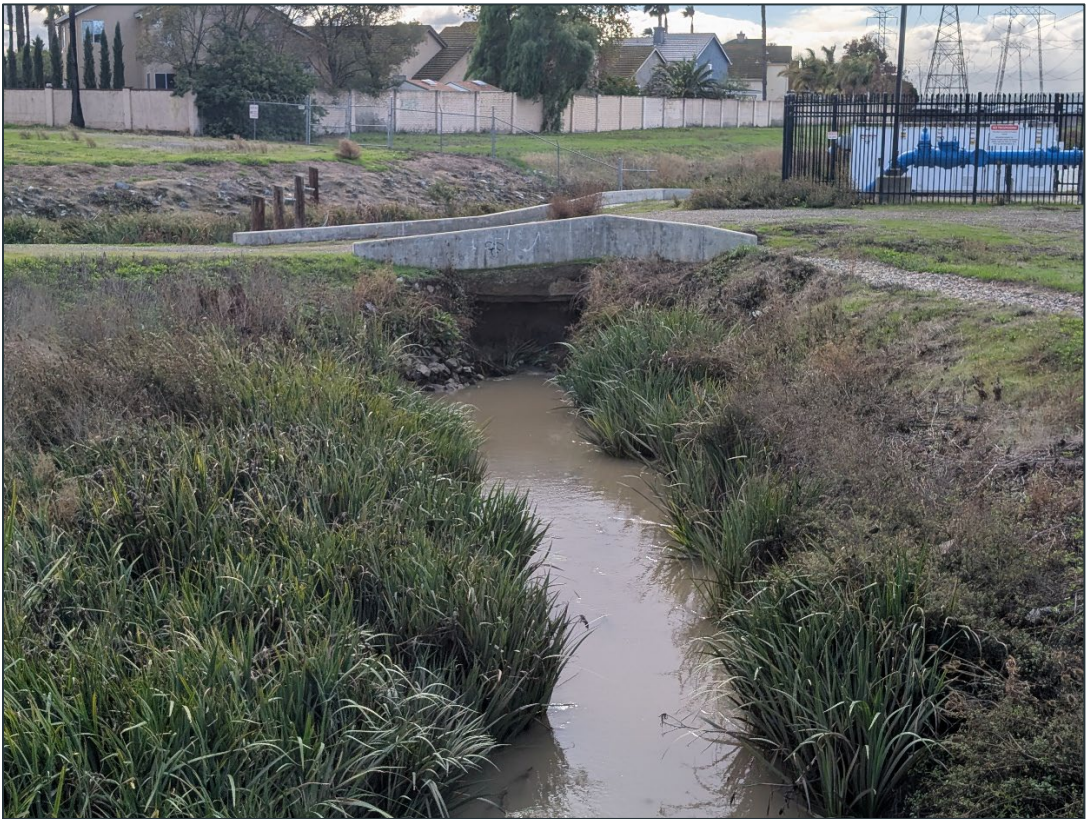
Figure 2: Erosion at Drainage Ditch Crossing
