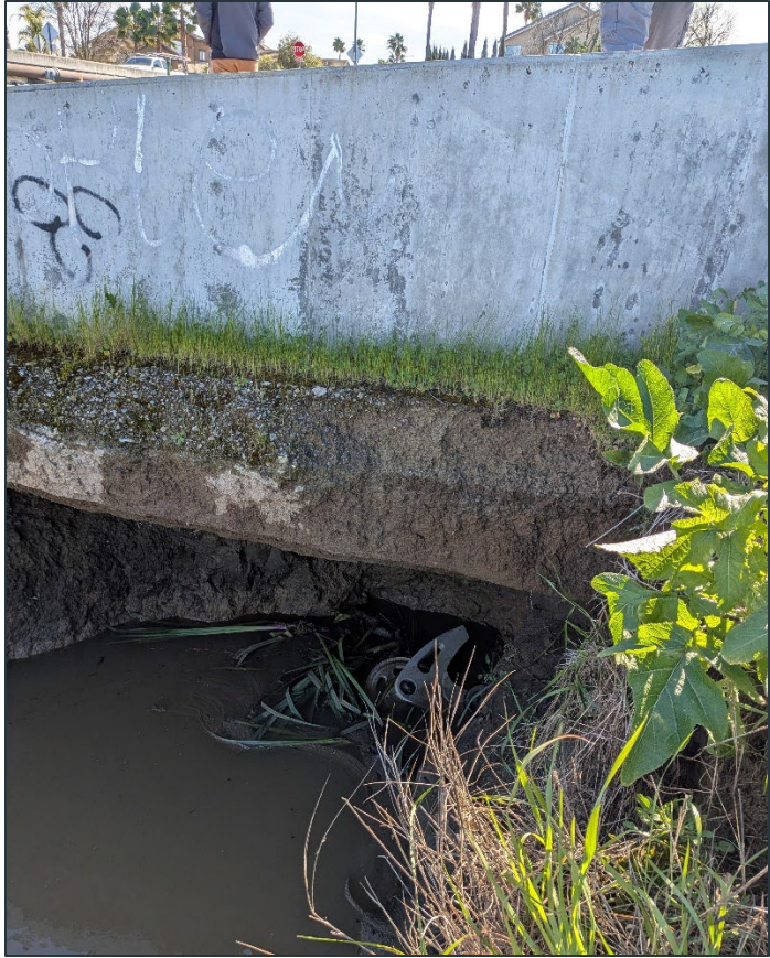
Figure 3: Erosion Undermining Beneath Crossing
