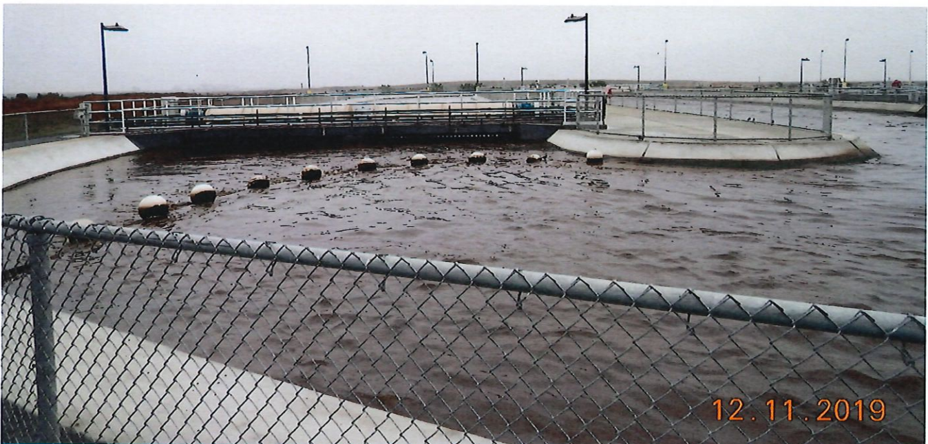
Figure 4: One of the two Oxidation ditches located in Plant 2 appeared in good working condition during the inspection.
