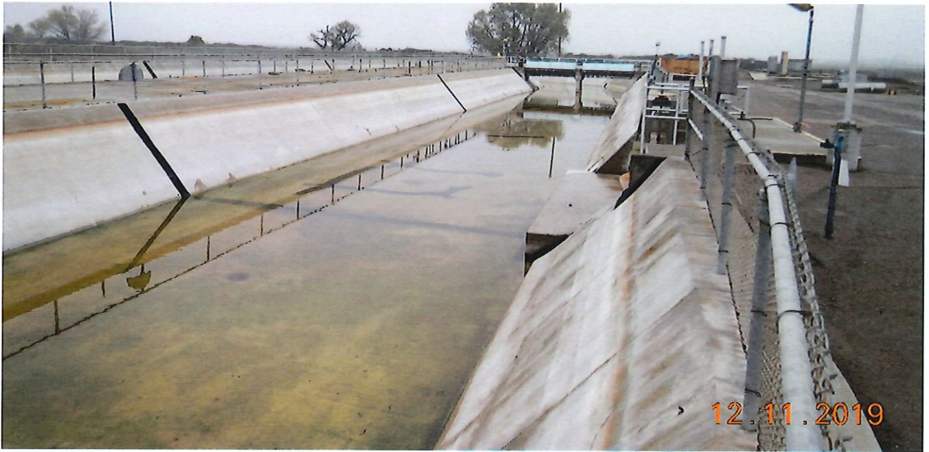
Figure 11: Oxidation ditch located at Plant 1. Currently, Plant 1 is not being used.
