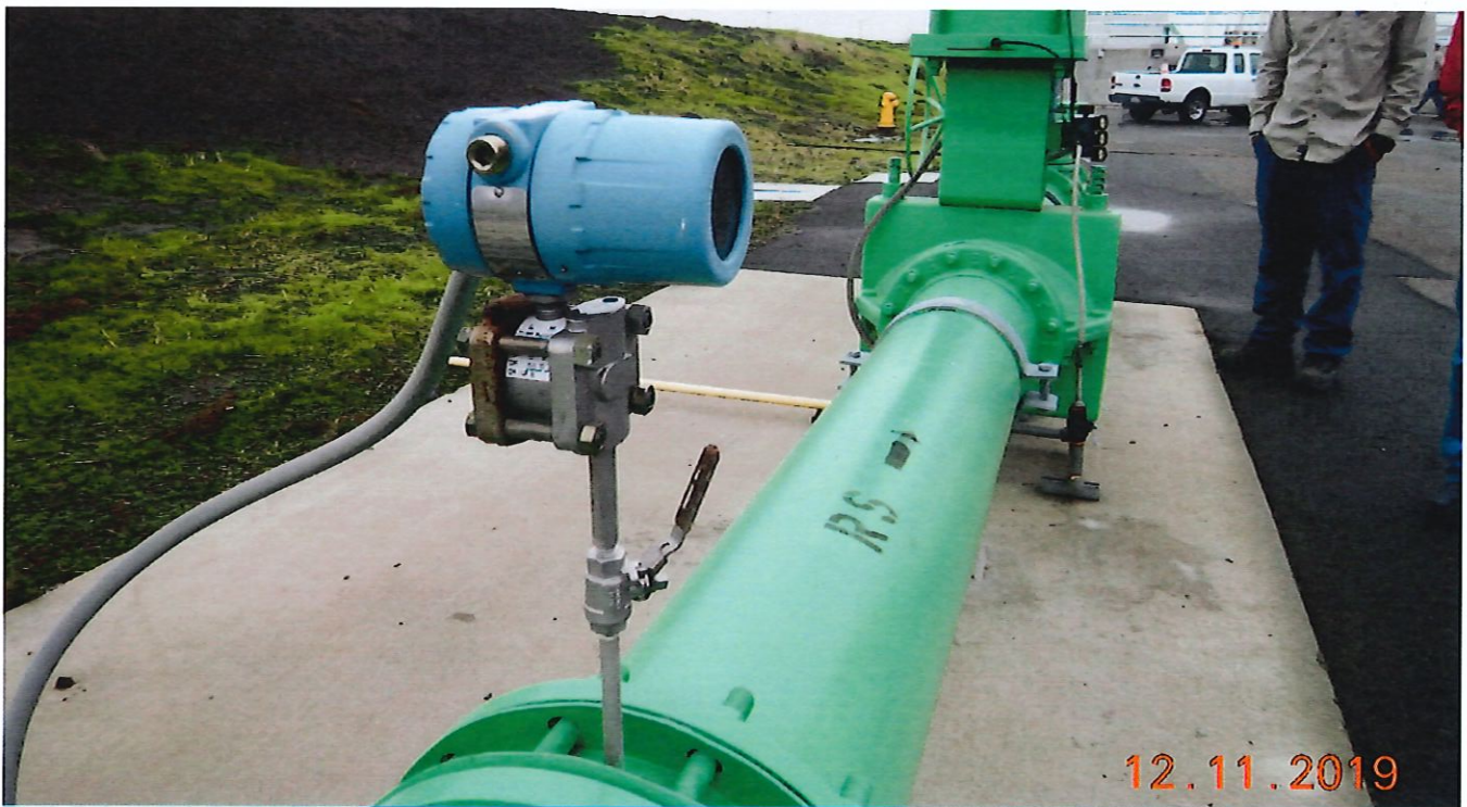
Figure 2: The Magnetic influent flow meter measures flow coming from Plant 1. The flow meter is used for internal process control and as a backup in case the Parshall Flume goes off-line.
