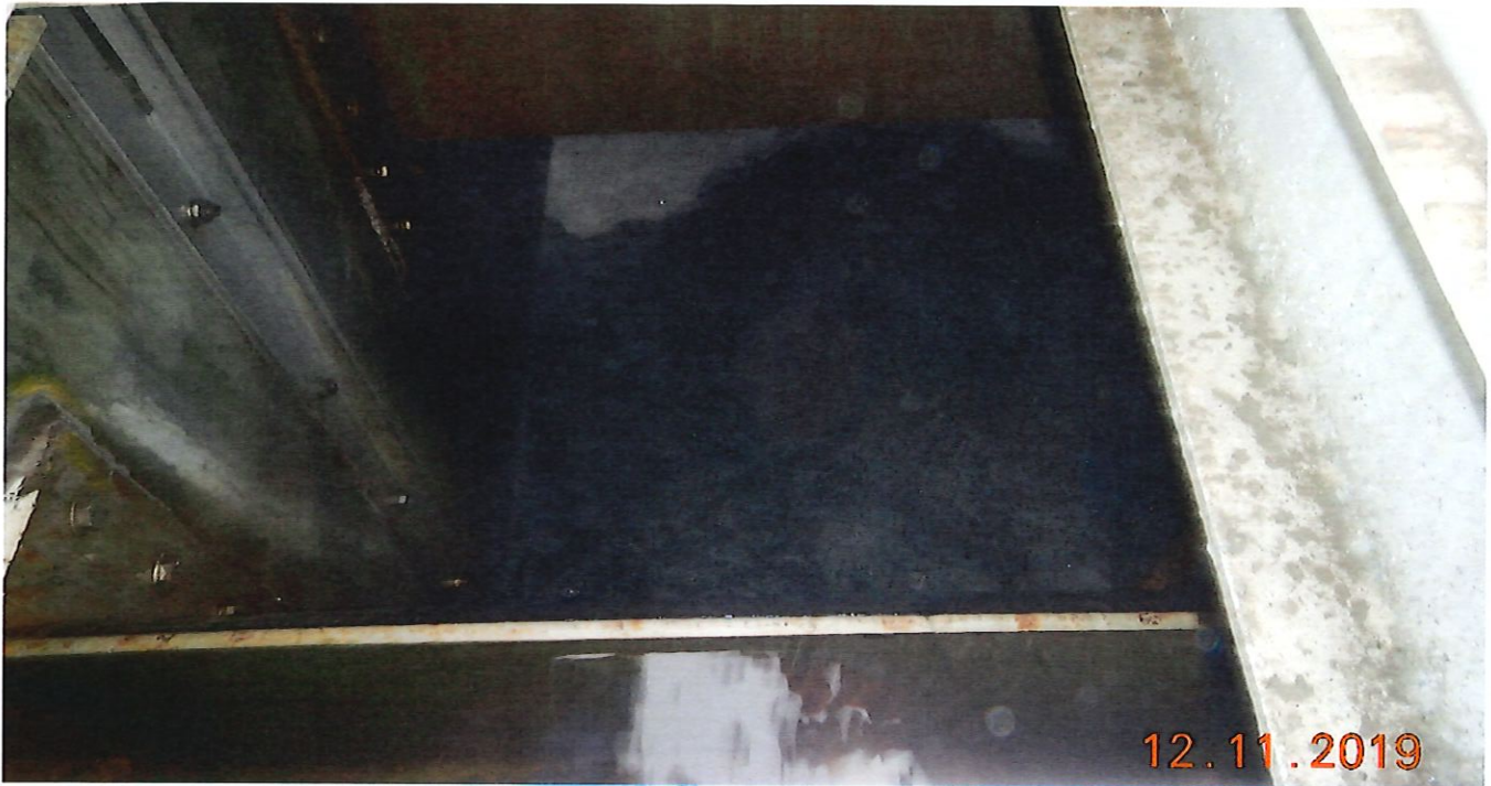
Figure 7: Inside view of one of the sand filters.
