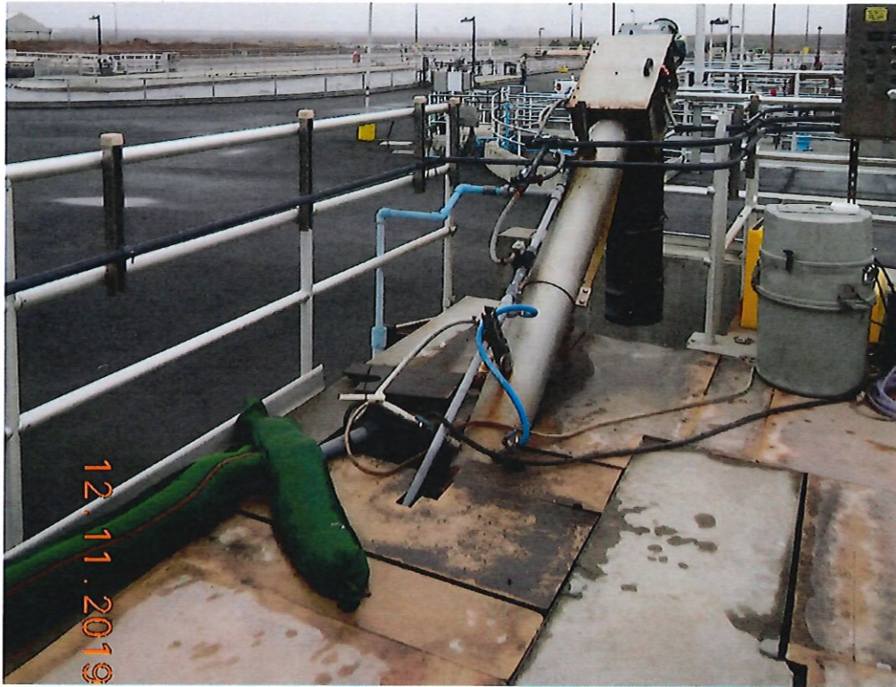
Figure 3: Mechanical grit removal located at the headworks of Plant 2 appeared in good working condition.
