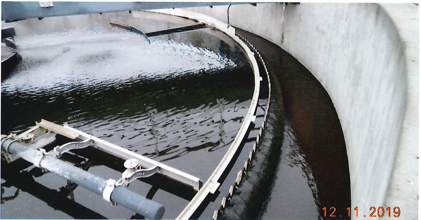
Figure 6: One of the three secondary clarifiers, located in Plant 2, appeared to be in good working condition.
