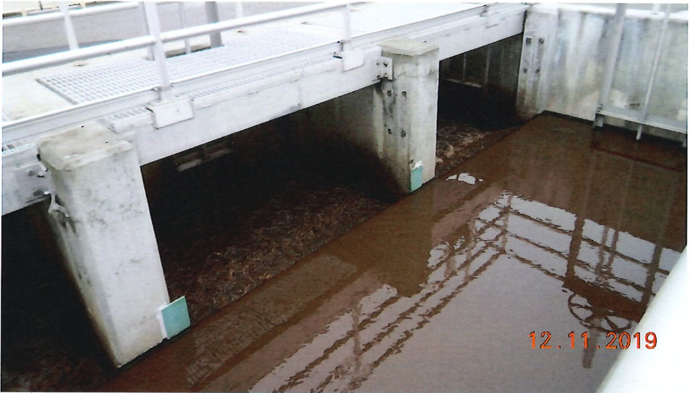
Figure 5: Splitter box located in Plant 2 which splits flow between three secondary clarifiers.
