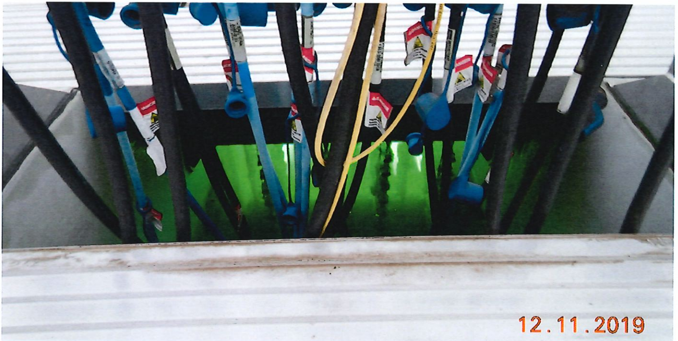
Figure 8: The Facility has two UV disinfection channels.
