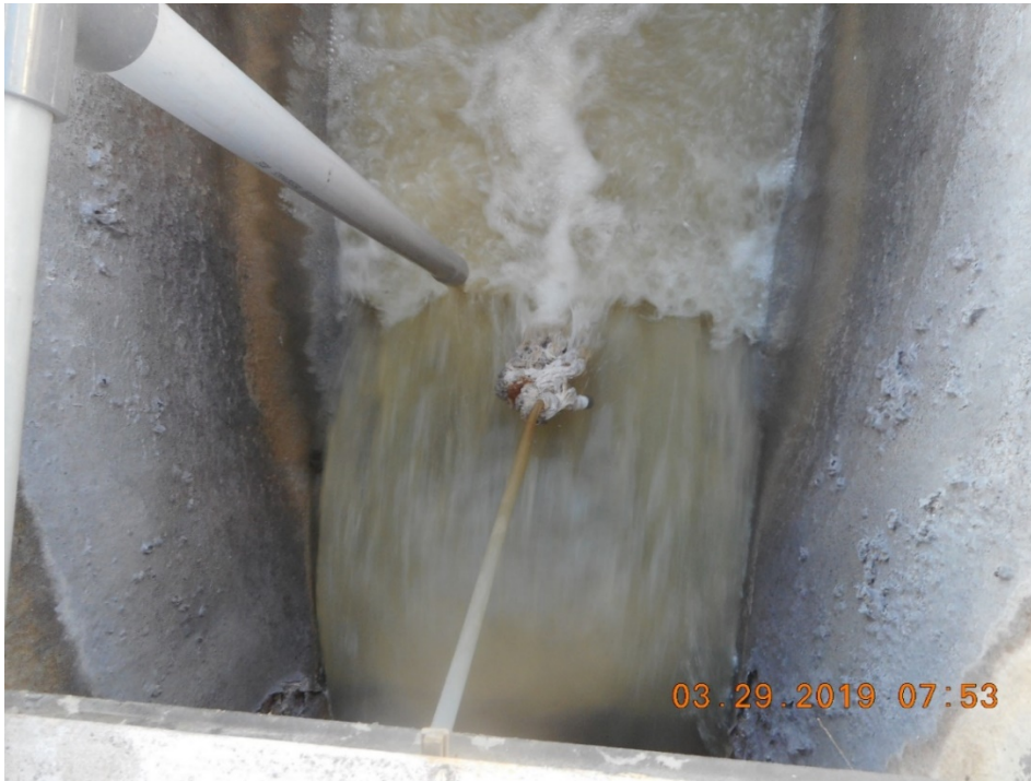
Figure 5-10 Portable Sample Intake Strainer Being Pulled Out of Flow Stream on 3-29-19
